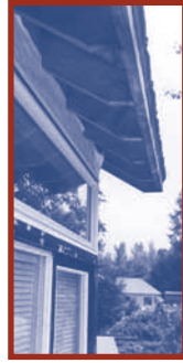
Open eaves, vents not screened (6 pts)
